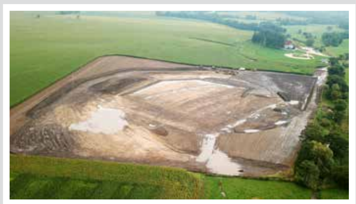
Shown above, rain once pooled on the Field of Dreams before Hydraway was installed. The new system diverted 2.5 inches of rain overnight before game day, allowing the field crew to mow the next morning.
